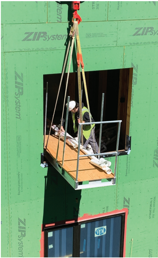
A load of PVC is lifted into place for unloading into a second-floor window at The Merin. According to Harvey's Plumbing's Mitch Rausch, the ability to get the right prefabricated assemblies to the right spot on the job provided a huge savings.
